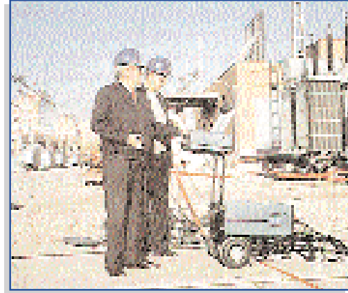
M4000 assembled for testing in the field
